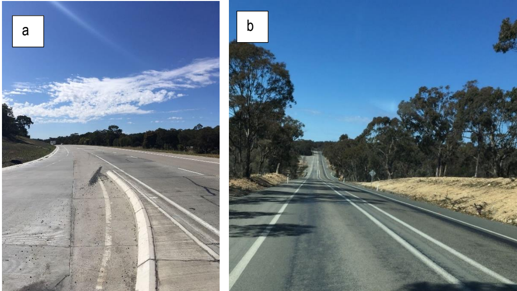
Plate 1 a) Intersection of Red Hills Road and Hume Highway b) Wide centre line on Brayton Road
